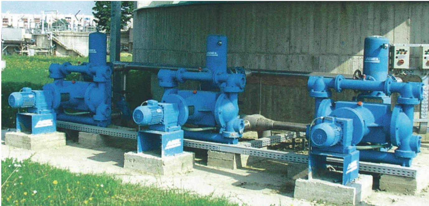
ABEL EM in a municipal WWTP – often the more economical alternative to transfer sludges with fibrous content
