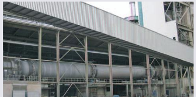
Cement industry – rotary kiln feed
