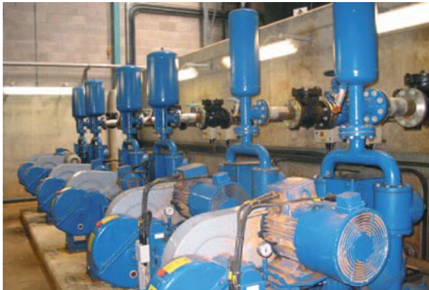
CM piston diaphragm pumps in a water treatment works in Northern Ireland
